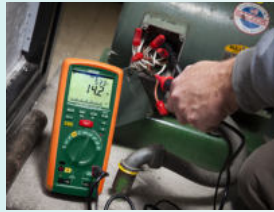
Insulation test on pump motor
